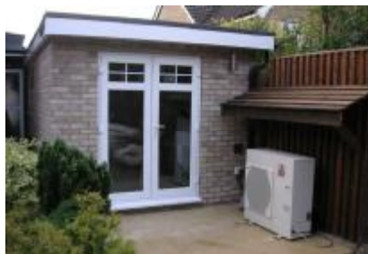
An 8.5kW Mitsubishi Air Source Heat Pump installed by GrEnergy
